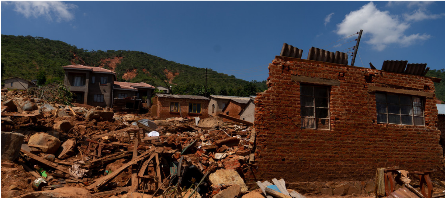
Houses damaged by Cyclone Idai: Ngango New Stands, Chimanimai - Zimbabwe. Severe weather events like cyclones have become much more intense as a result of climate change.
